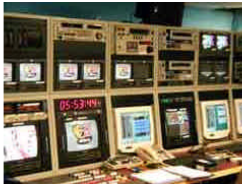
master control - KWBM
