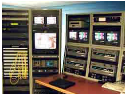
master control - KWBM
